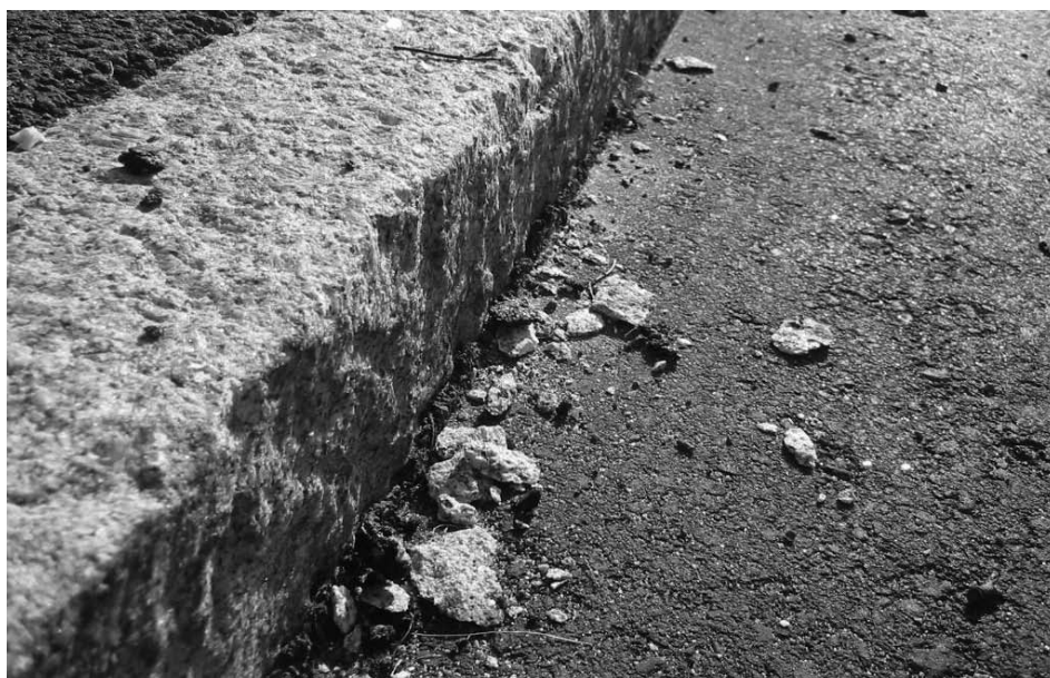
Figure 1: Kerbstone damaged shortly after installation, most likely due to poor resistance to mechanical impact. A property not included in the product standard.
